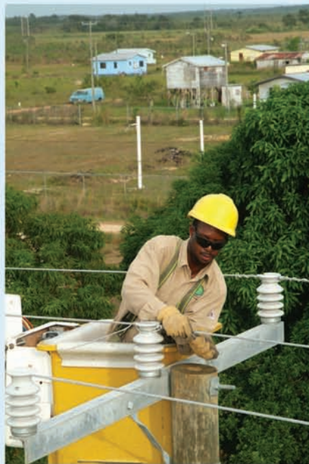
In 2006, BEL carried out numerous projects under its Capital Investment Program aimed at system improvement and expansion. Above, work being carried out on the distribution line in Hattieville.
