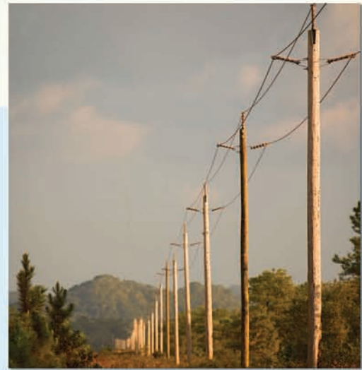
Southern Transmission Line upgraded to 69kV from 34.5 kV in 2006.
